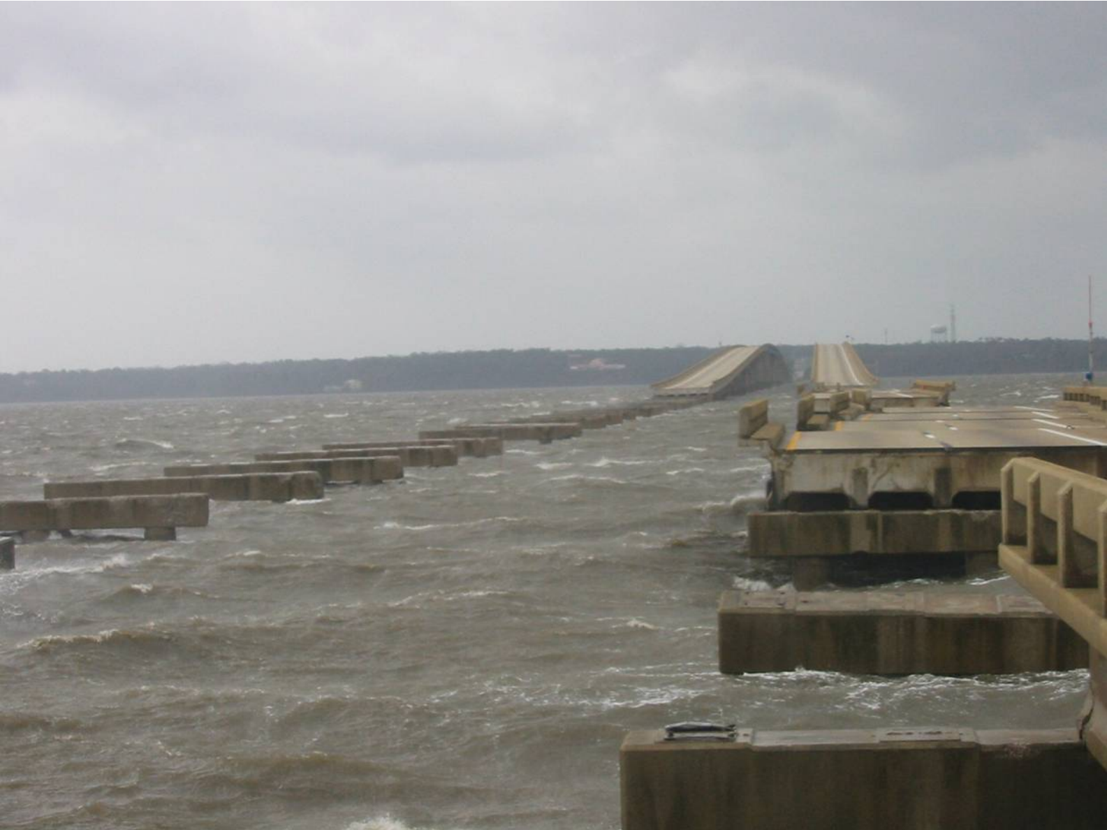
Figure 3 I-10 Bridge after Hurricane Ivan
